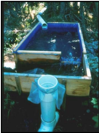
AWA's "low drop, high flow" hydroelectric system. (Photo courtesy of Kirk Hoessle)
