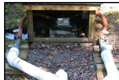
Hydroelectric system turbine (Photo courtesy of Kirk Hoessle)
